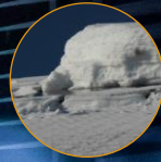
Heavy snow load frame
